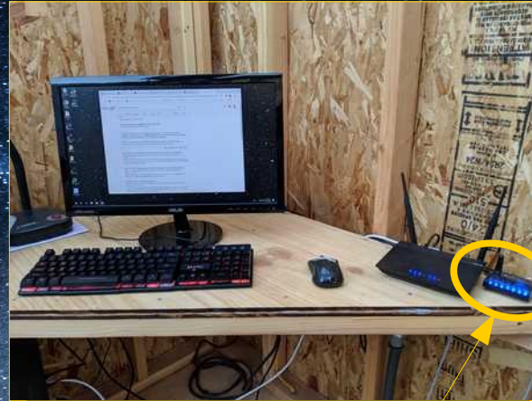
Wireless Receiver / Access Point
