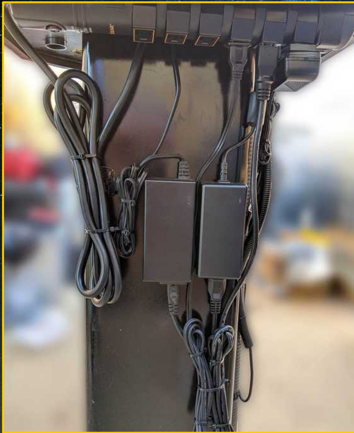
12Volt DC Power Bricks
