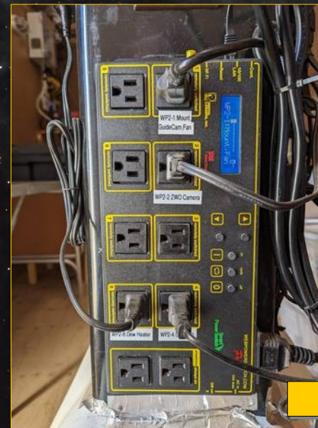
Pier Power Distribution (WP2)
