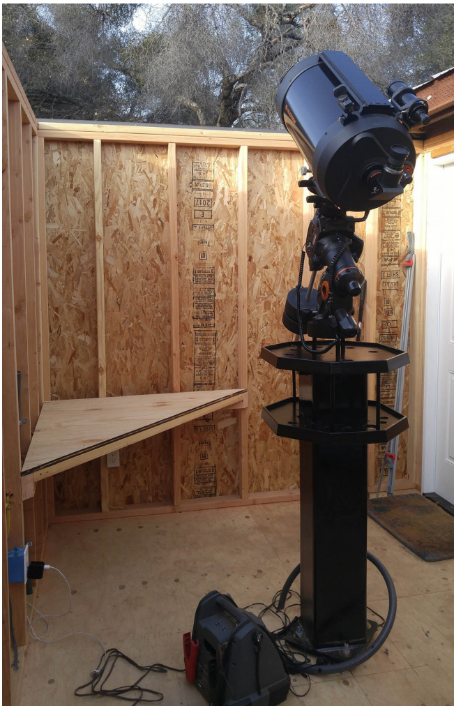
Pier Shelves and Computer Desk (Note Temporary Mount Power Supply and conduit to PC Desk)
