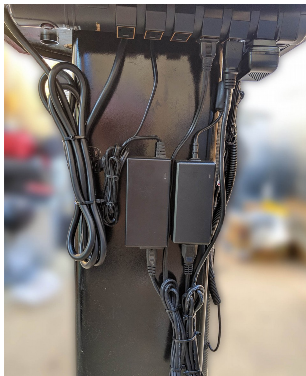
Pier North Side With Power Strip (Top) and Adhesive-Mounted Power Bricks
